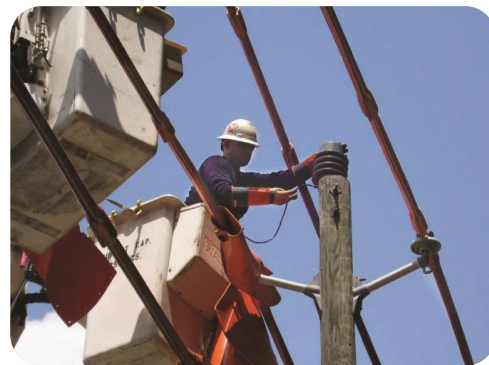
Figure 5: North Carolina Installation
